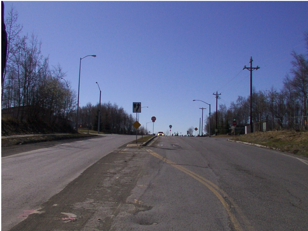
Near 100 th Ave, the grades approach 8% and sight distance is poor.
