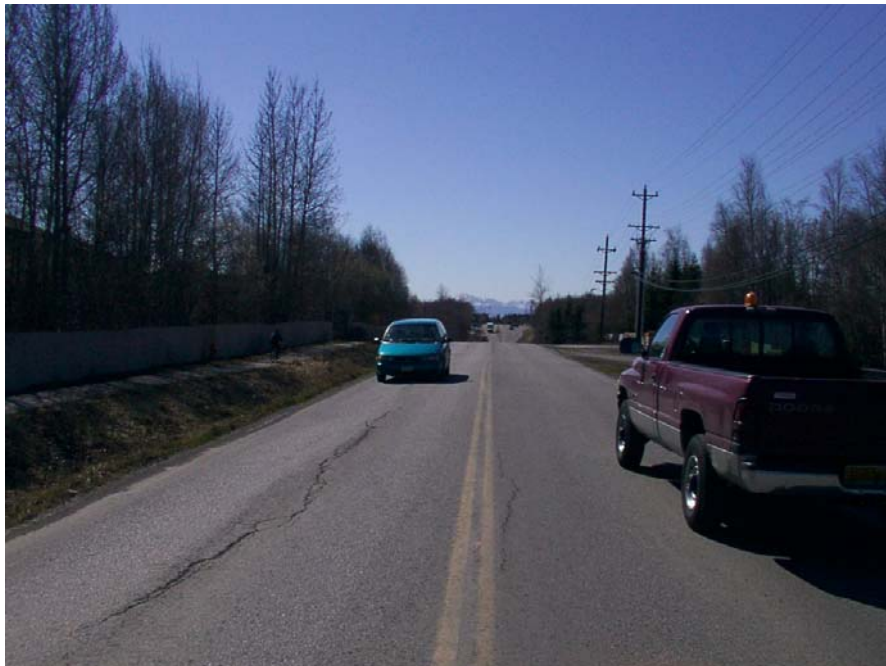
The existing pavement is in poor condition with numerous cracking.
