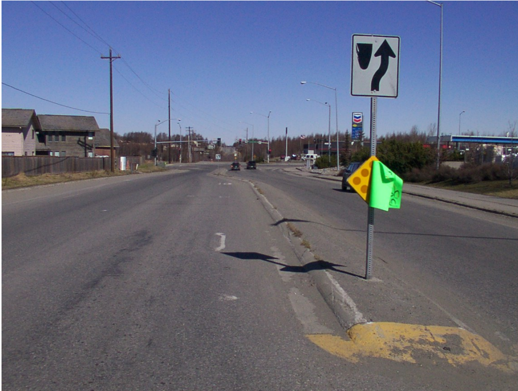
Near Dimond Blvd., Existing curb & gutter, a narrow raised median and auxiliary lane.
